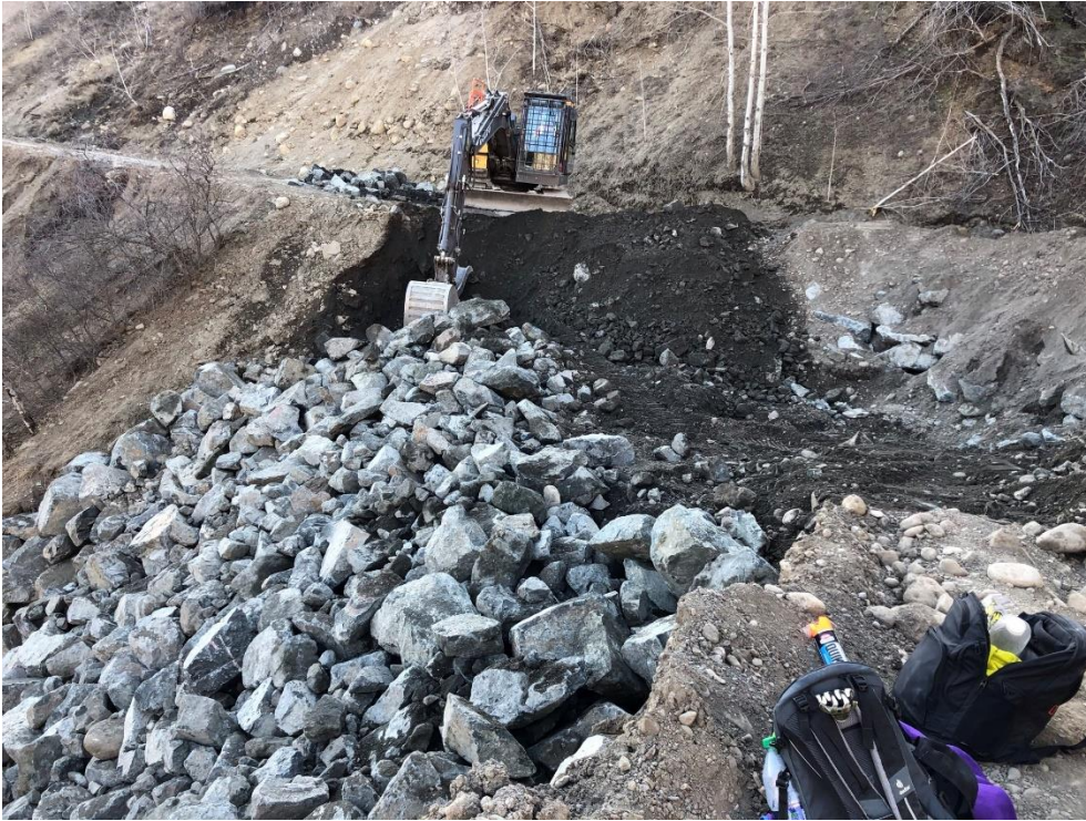
Highway 51 washout near Telegraph Creek, BC, April 14, 2021. Photo credit: Emergency Management, British Columbia
